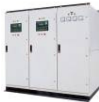
DSE-550 Parallel Control Panel system
